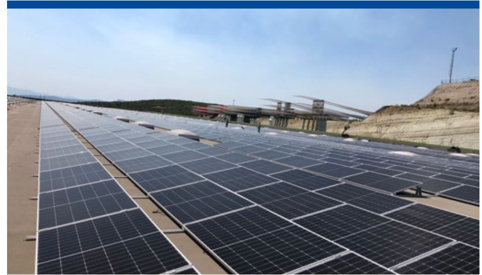
Solar panels in Türkiye.
